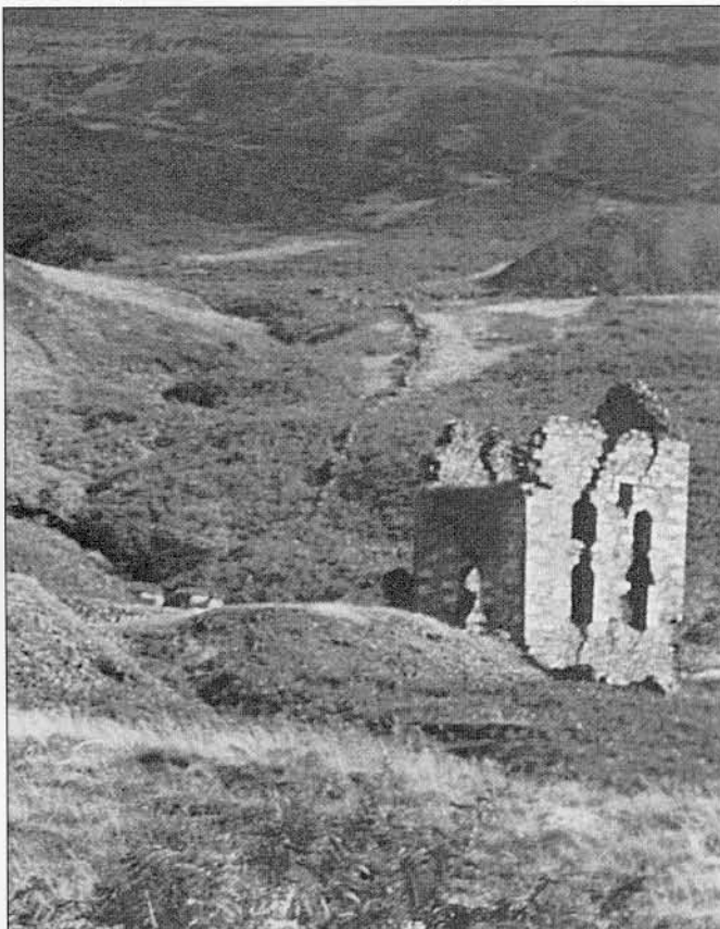
Plate 1. Pibble Mine Cornish Engine House during the 1950s showing the collapsed bob wall and large cracks on the west elevation. (Source Creetown Local History Museum).
